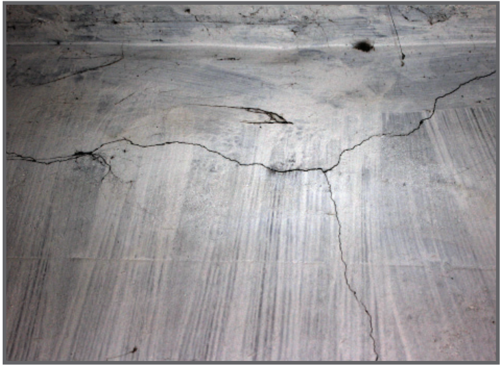
POST-TSUNAMI HOUSING IN PERUMBAKKAM, CHENNAI: CRACKS IN THE FLOOR
