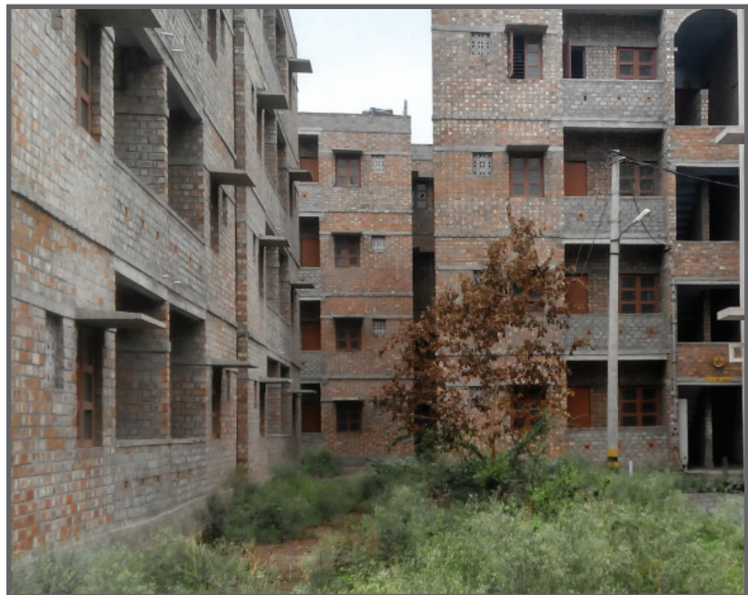
DETERIORATING CONDITIONS AT BAPROLA RESETTLEMENT SITE, DELHI
