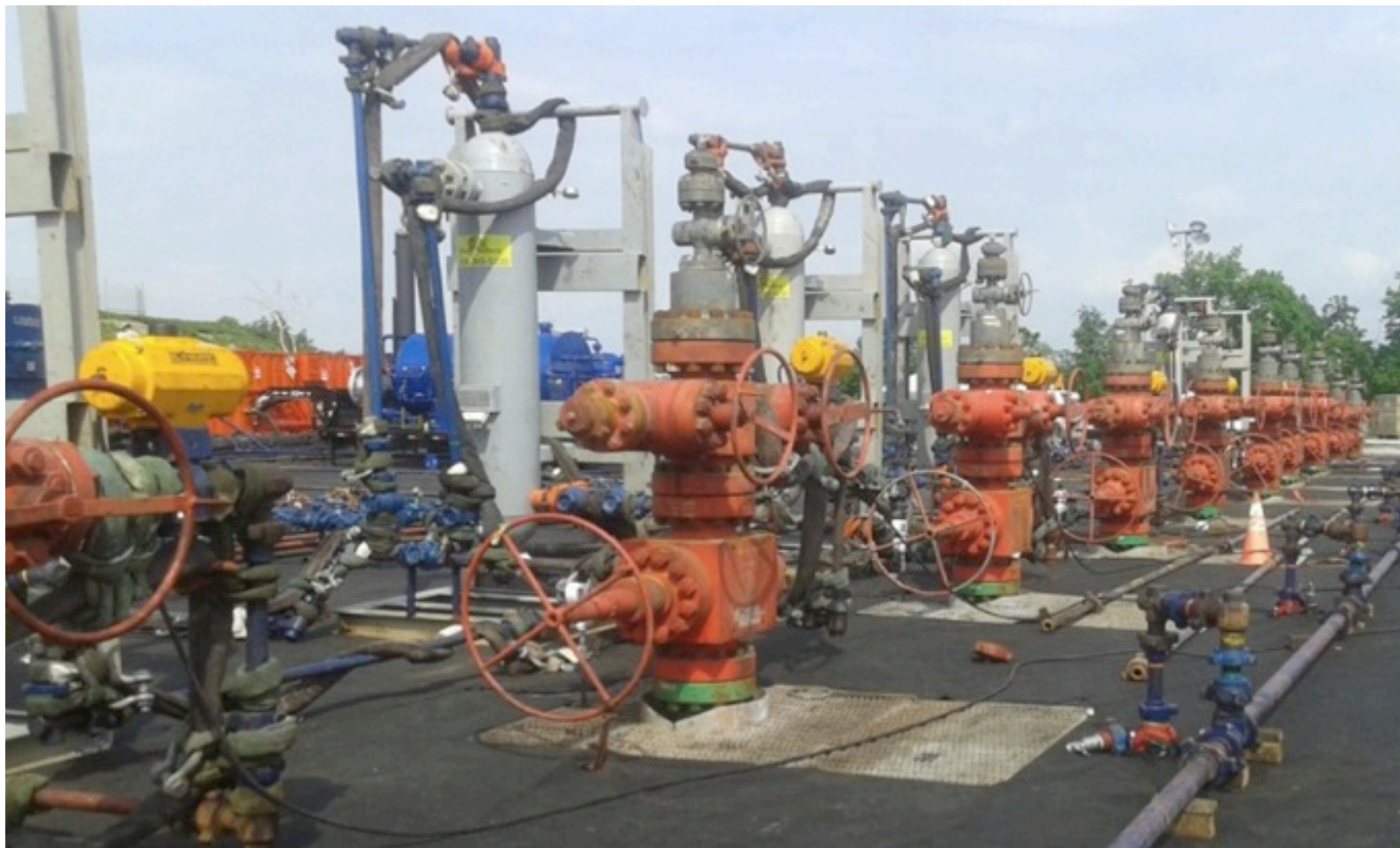
Figure 7: A single well pad may have up to 11 or 12 different wells drilled; in this picture the red Christmas tree-like valves close off each well drilled. Ten are visible in the image. Photo: JDTaillant, at a Pennsylvania-Marcellus Shale gas well.
