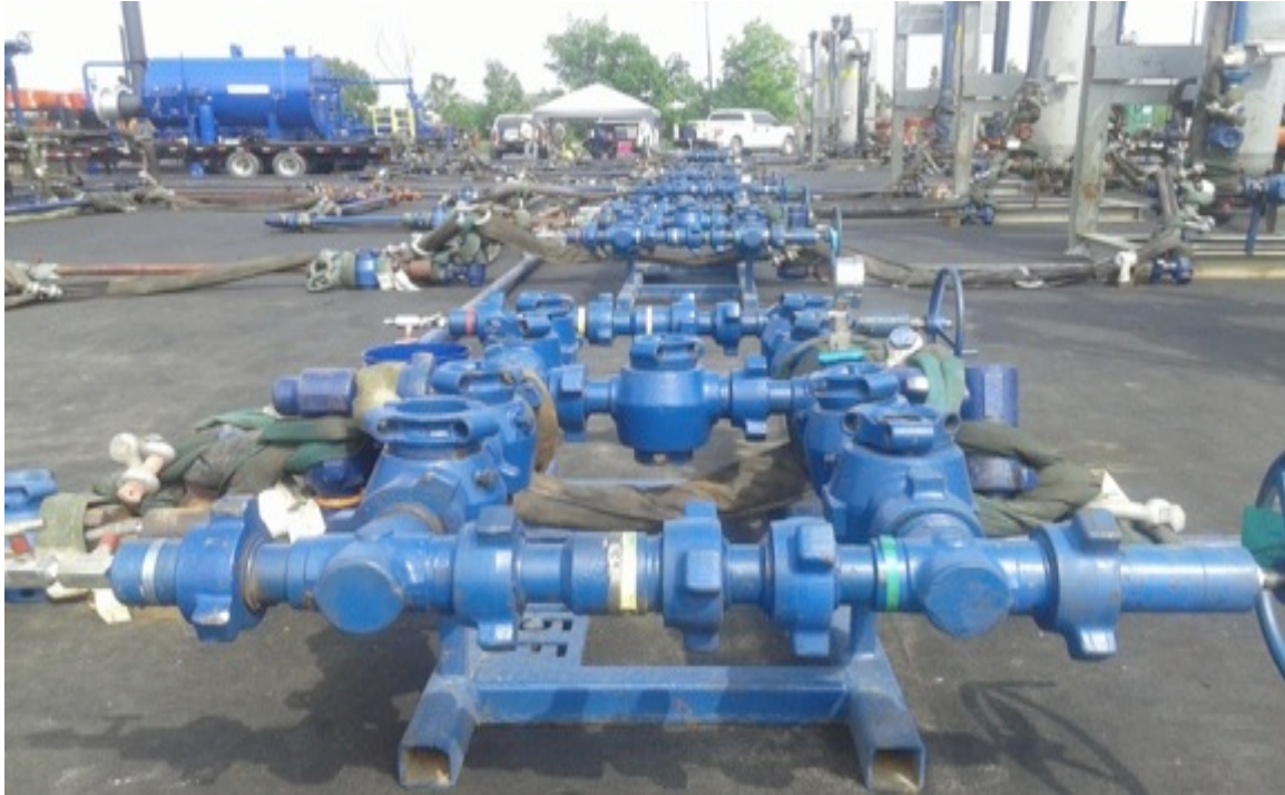
Figure 17: Thousands of joints in fracking pipe unions are potential points of methane leaks. Photo: JDTaillant
