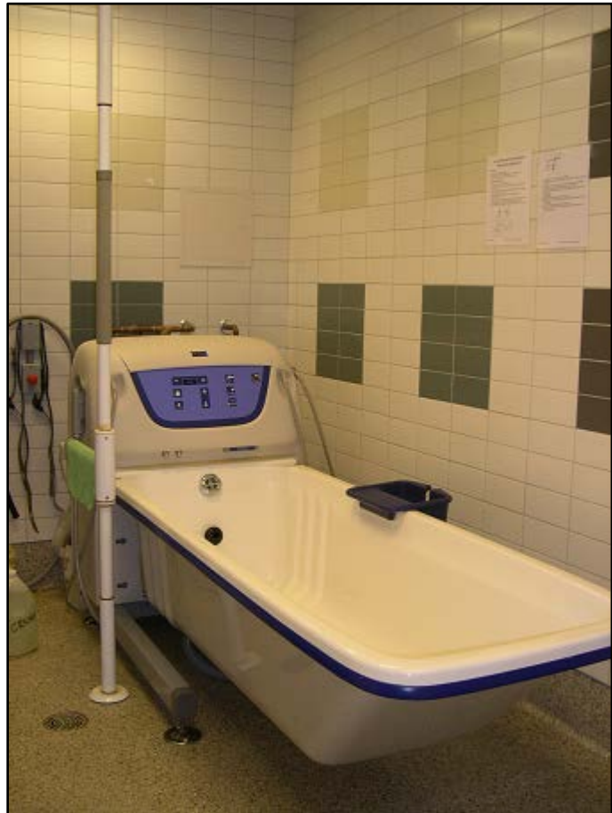
Pacific Regional Treatment Centre: Arjo Tub
