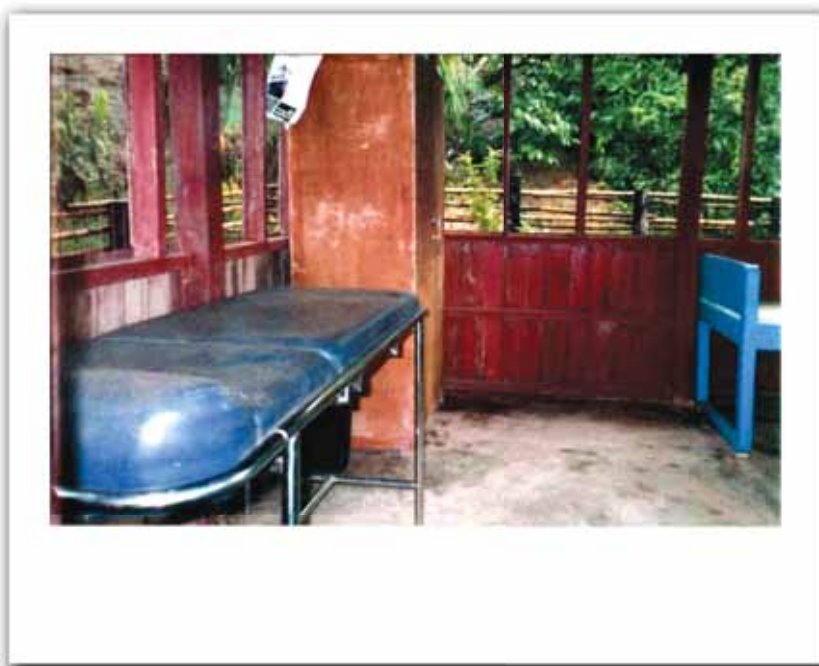
A Total health clinic in the pipeline corridor in disrepair, photo in 2009 © EarthRights International, 2009
